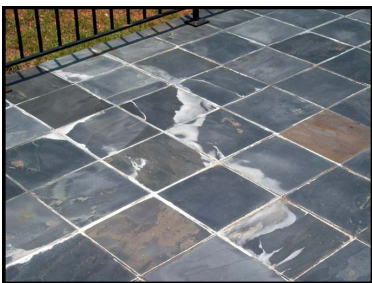
Efflorescence on Tile
